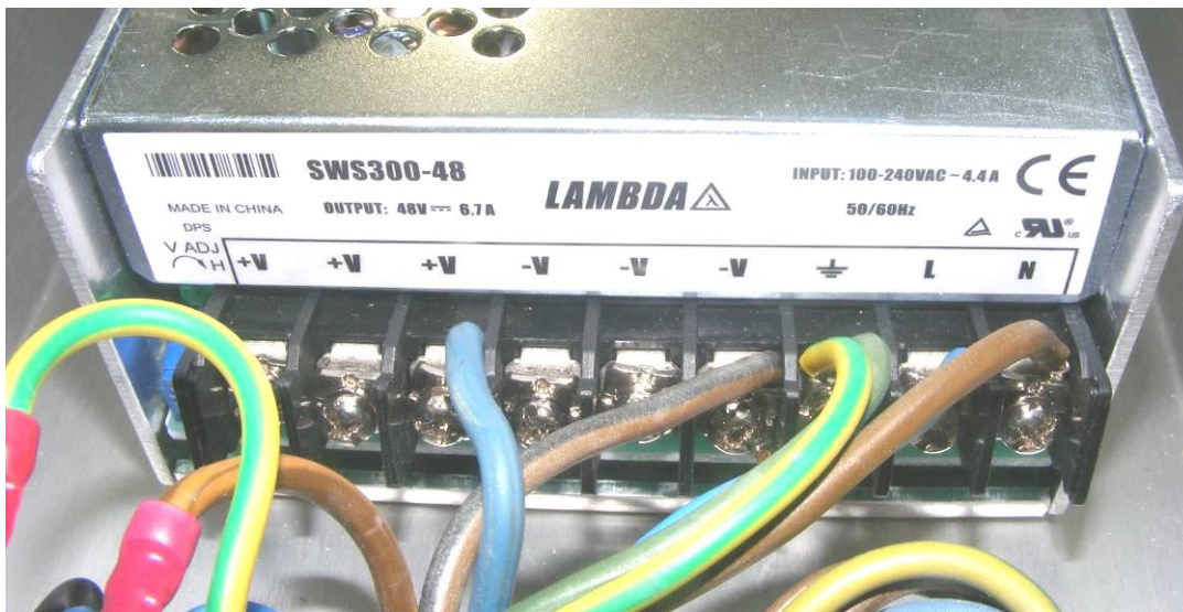
Power supply internal connections
