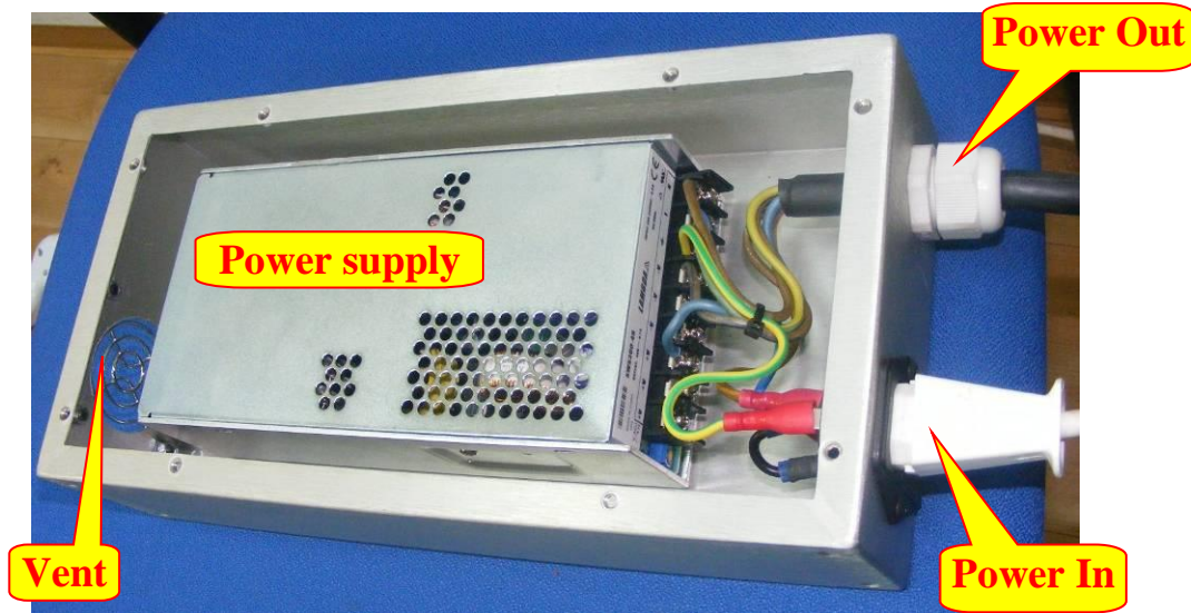
Power Supply (cover removed)
